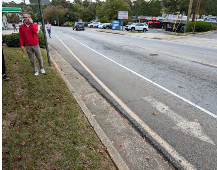
Bike lane pavement markings are faded and do not have clear visibility.
