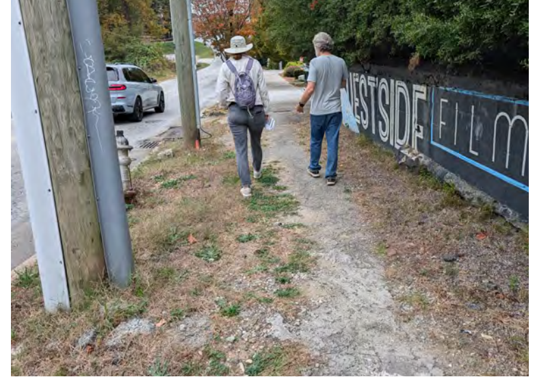
Gaps between paved sidewalks have clear desire paths from foot traffic. These paths are uneven and present hazards and barriers for users with mobility challenges.
