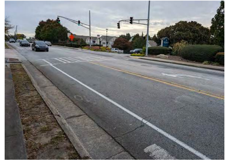
Crosswalk near Willowest in Collier Hills apartment complex road intersection is faded and doesn't appropriately intersect with the bike lane.
